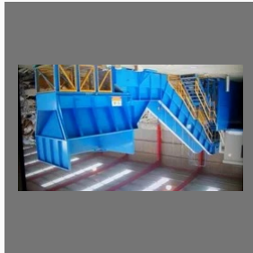
Pneumatic Conveying System
